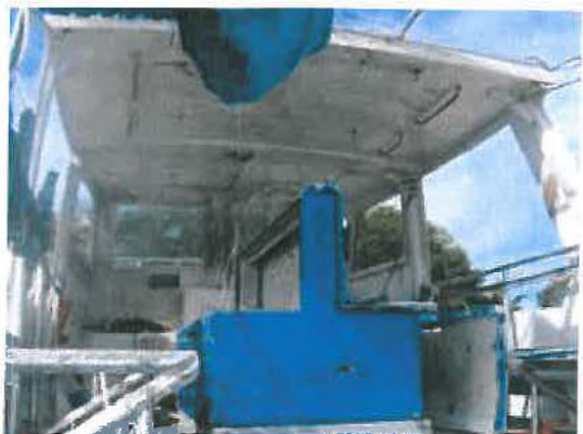
View of engine hatch cover. The hatch cover moved forward, under the bimini as the vessel sank.
