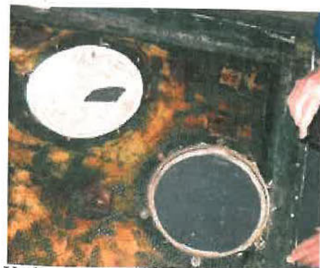
Underside of engine compartment deck plate, no gasket or sealant visible.
