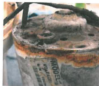
Visible corrosion. Making it likely that the pump had been inoperable for some time, possibly after the failed attempted self repair.
