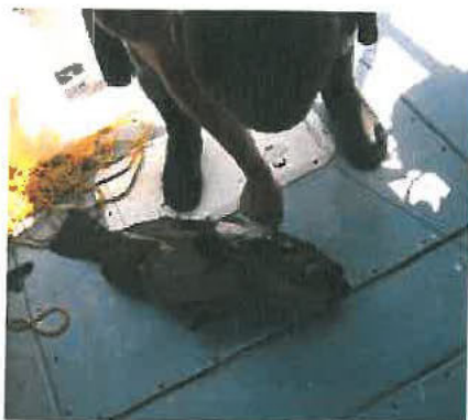
Unsecured deck plates. A single screw is visible on the lazarette deck plate.
