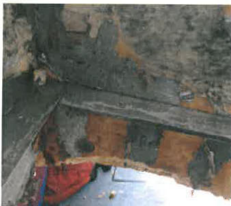
Interior wet rot and decay of the engine hatch cover.
